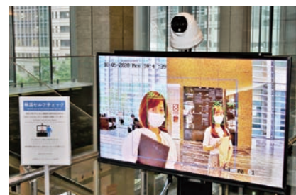
Monitor installed near the entrance of the head office building to measure the body temperature of people entering.
